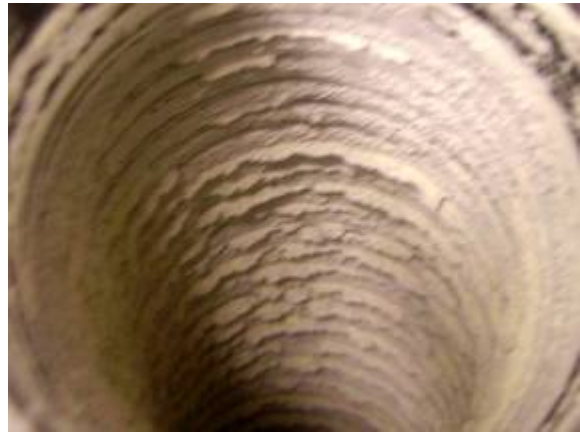
Clogging of flexible suction arm after 20 kg solder
